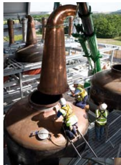
Stills being installed at the new Roseisle distillery in Speyside
